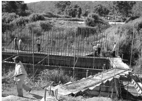
Fig -11 The type of a access bridge which was constructed to the widening works of the box culvert
