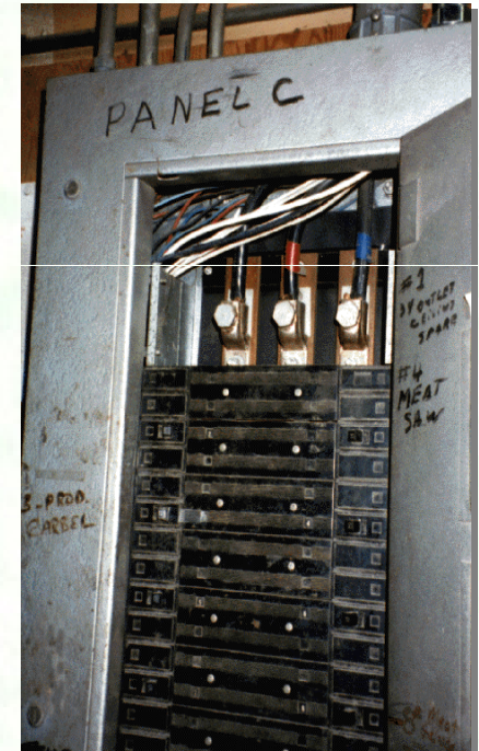
Exposed live circuits
