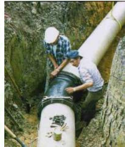
Needs a trench box
